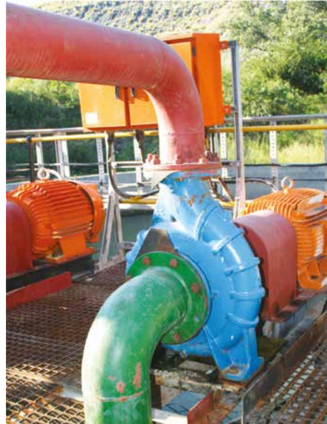
NT Pump Station
