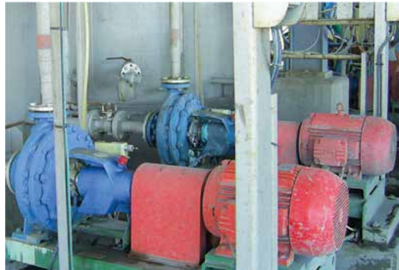
Platinum Mine - Acid plant
