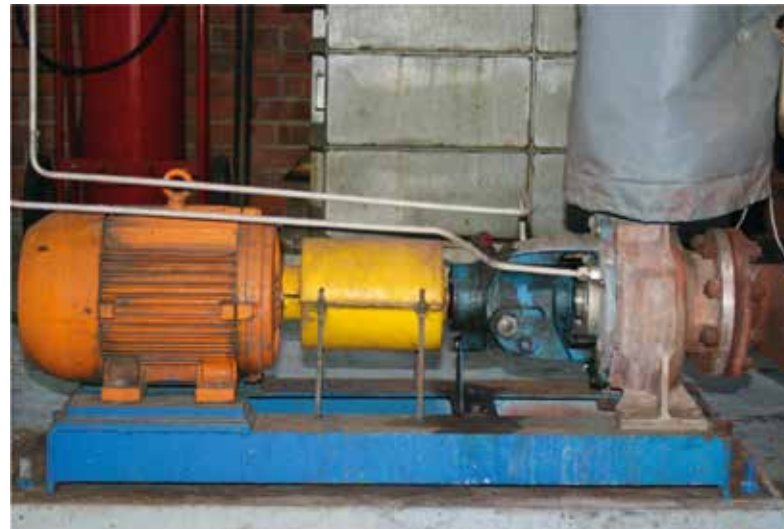
Platinum Mine with a flushed mechanical seal arrangement
